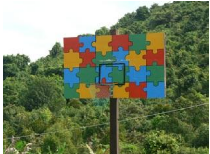
building a second sandpit, painting sandpits bright colours, erecting jungle gym, erecting and painting competition size basketball ring and backboard
